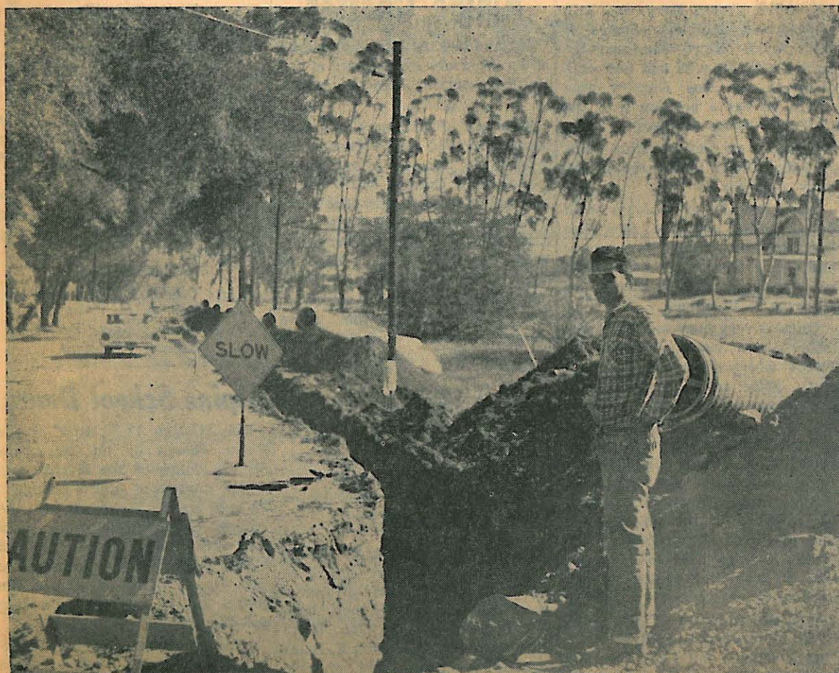
Water line at Arnold Way and Tavern Road being inspected by Mr. A. L. Adams, President of the Alpine Heights Municipal Water District and Director of the Rio San Diego Municipal Water District. The first parsonage built in Alpine in 1892 showing in right background. Bea LaForce Photo
